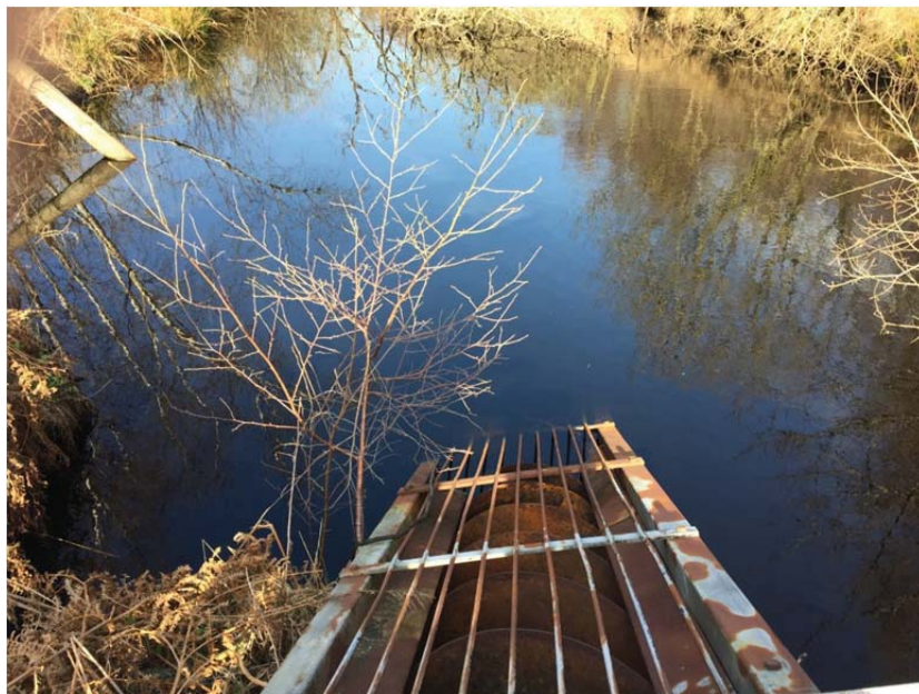
Image 2-2: Mulgeeth – Screw Pump Blockage
